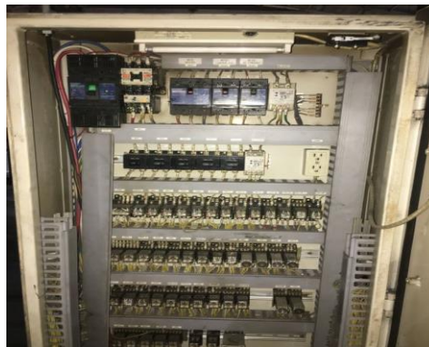
Gambar 16. Panel Listrik Flashbutt
