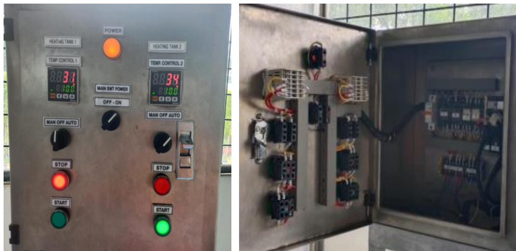
Gambar 4. Panel Kontrol Killing Tank Mode Steam (Sumber : PT. Kalbio Global Medika)
