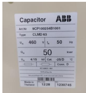
Gbr. 7 Data kapasitor bank
