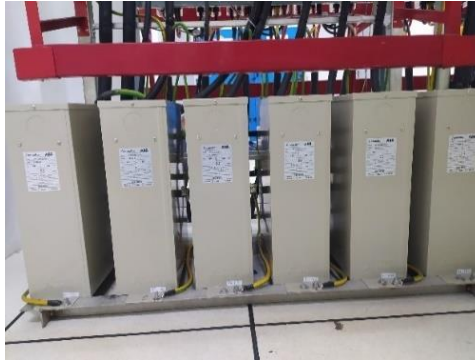
Gbr. 3 Kapasitor bank shunt
