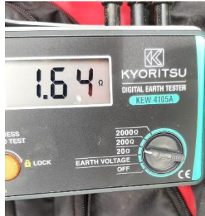
Gambar 6: Nilai Hasil Pengukuran Pentanahan Tower 64
