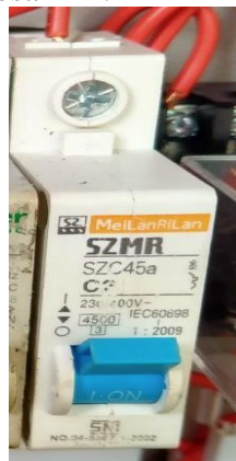
Gambar 19. Miniature Circuit Breaker (MCB) 2A
